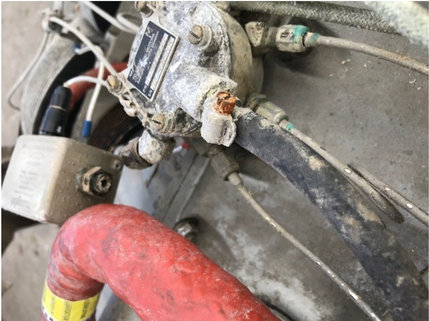
Photo 3 – View of broken fuel flow sensor line
