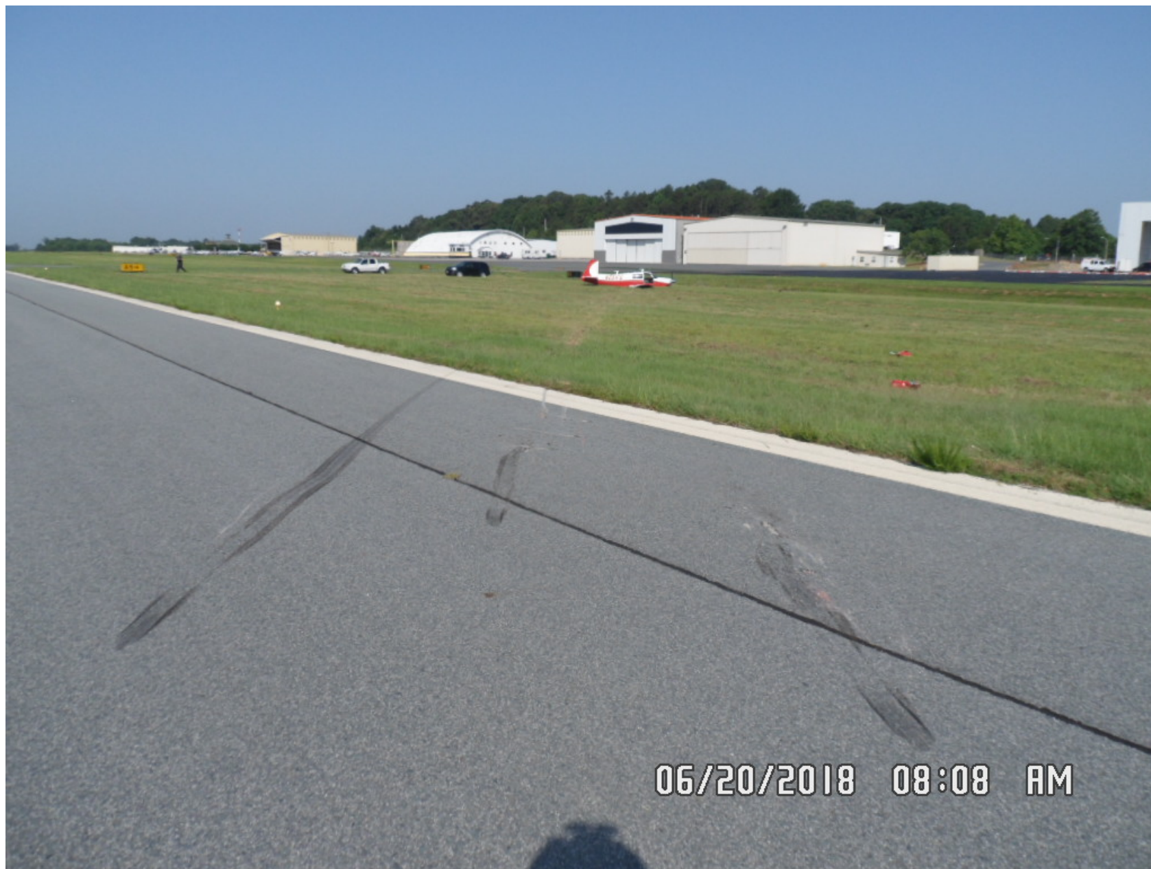
Photo 1 – View of Initial Ground Scars on Runway 23 (FAA)
