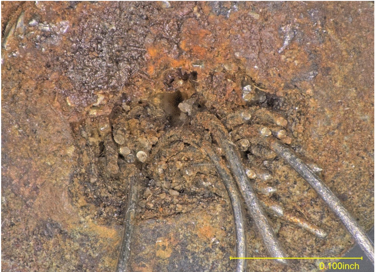
Figure 3 – Closer view of the fractured wires from the cable bundle in Figure 2, as received.
