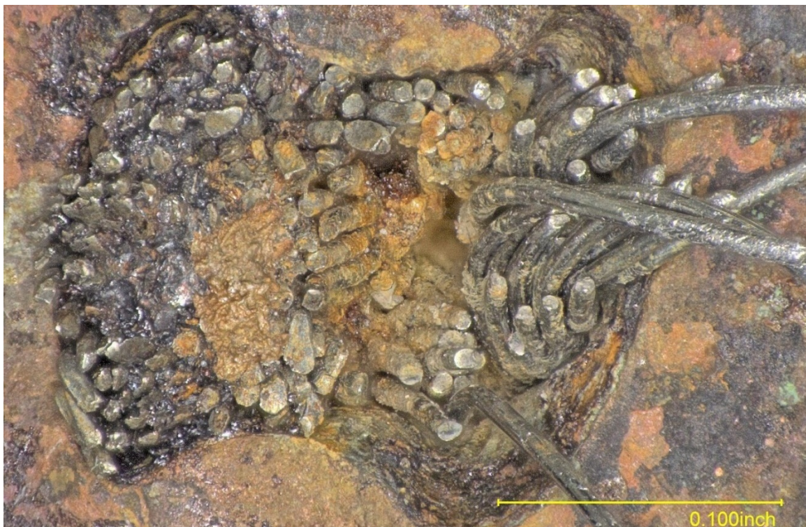
Figure 5 – Closer view of the fractured wires of the cable bundle, after cleaning.
