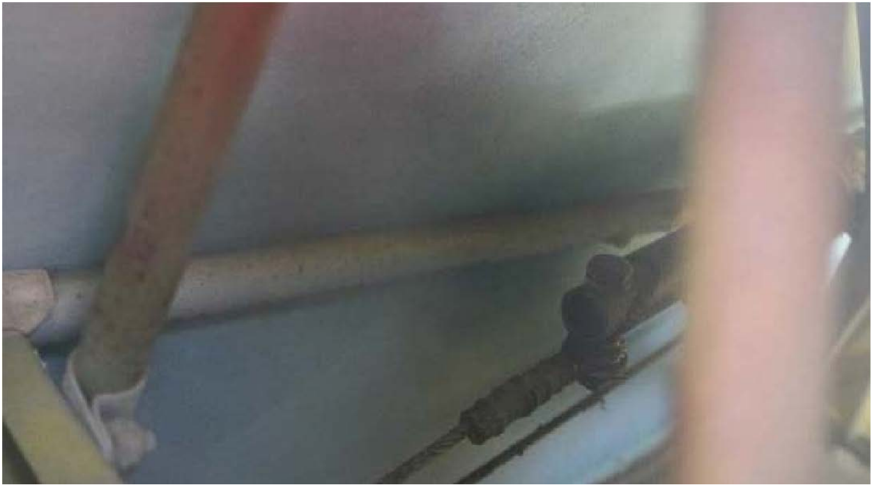
Figure: FAA Digital Photograph. View of the nicopress sleeving for the elevator flight control cable. Note there is no visible cable protruding from the nicoproess afer it made its loop through the control horn fitting.
