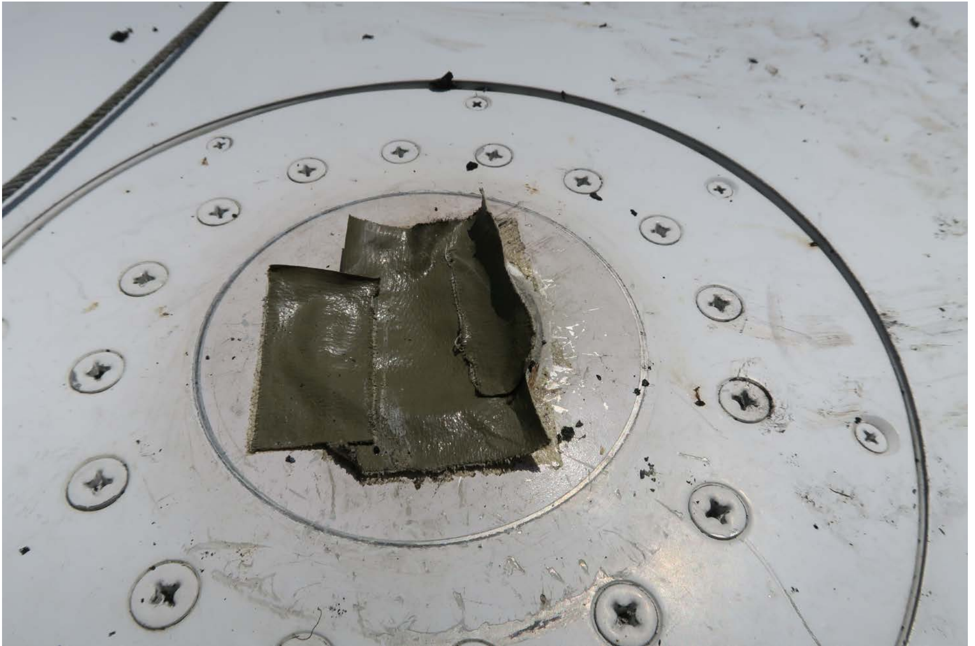
Photo 9 – Close up view of tape over right fuel port filler showing some heat damage
