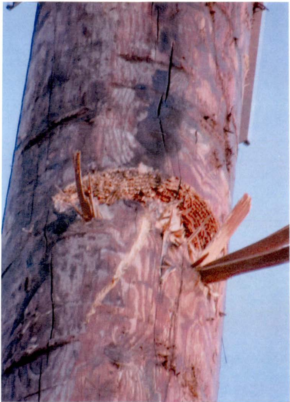
Damage to B Pole Structure 15884
