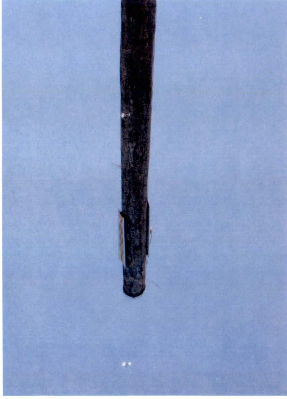
22 B Pole Structure # 15884
