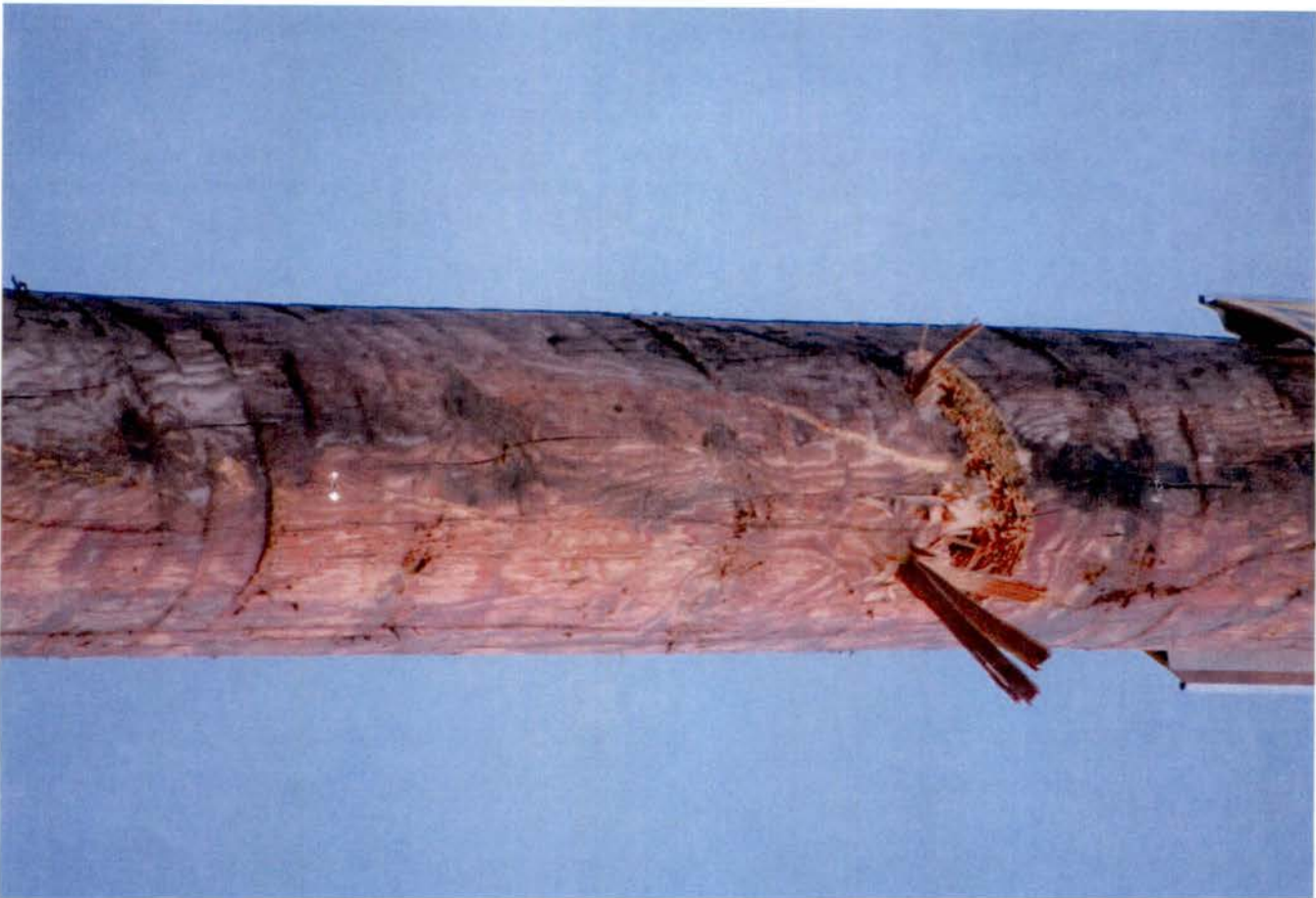
71 B Pole structure # 15884
