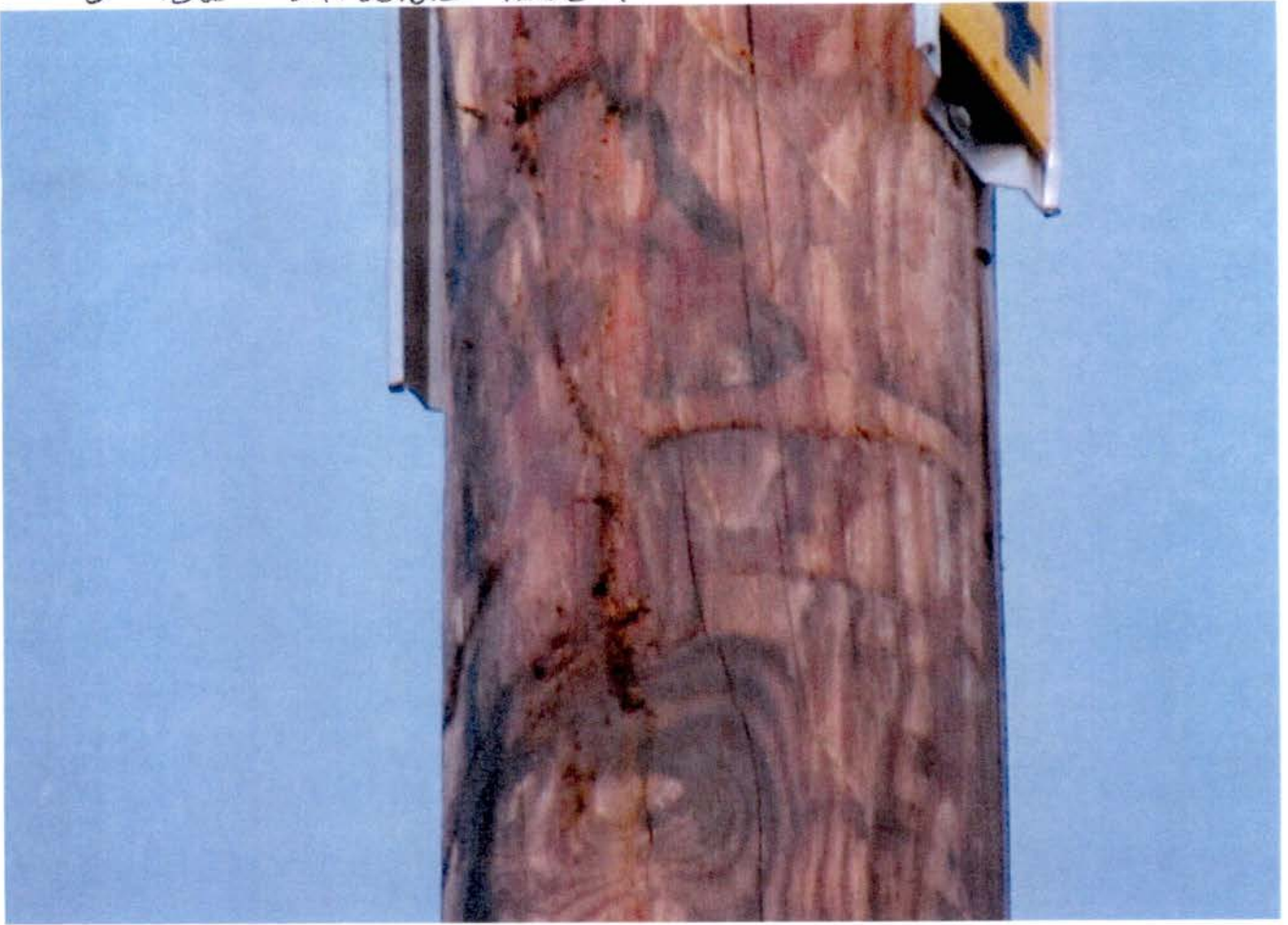
B Pole Structure 15884
