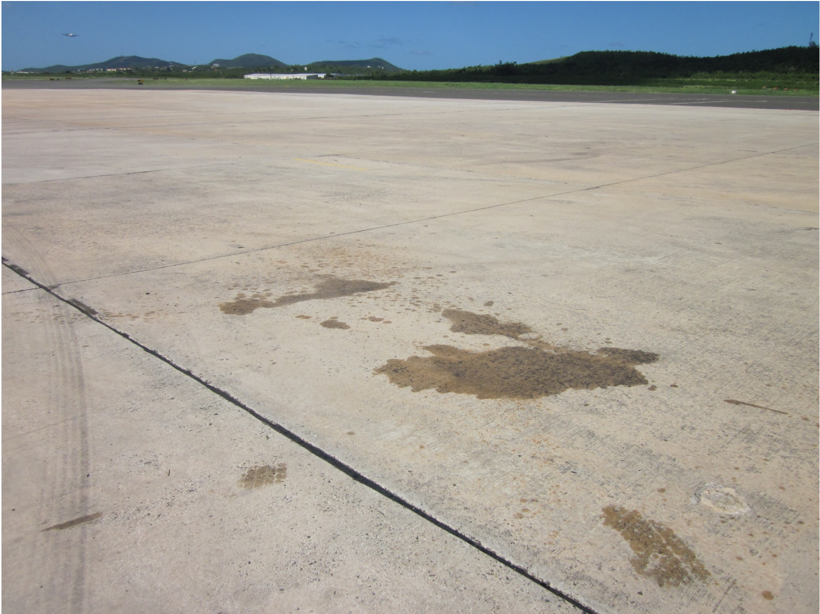
Photo 7 – Stain on the ramp where N4484A was parked. (Photo courtesy of the FAA)
