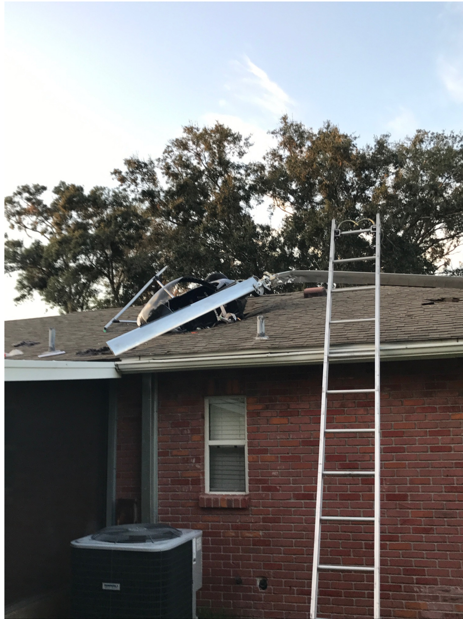
Photo 3 – Left Side View of main Wreckage – Courtesy of FAA
