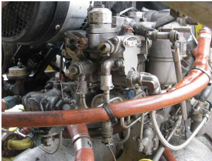
Photo No. 16 Py line at the fuel control unit
