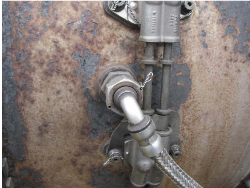
Photo No. 45 One of the ignitor leads at the gas generator case
