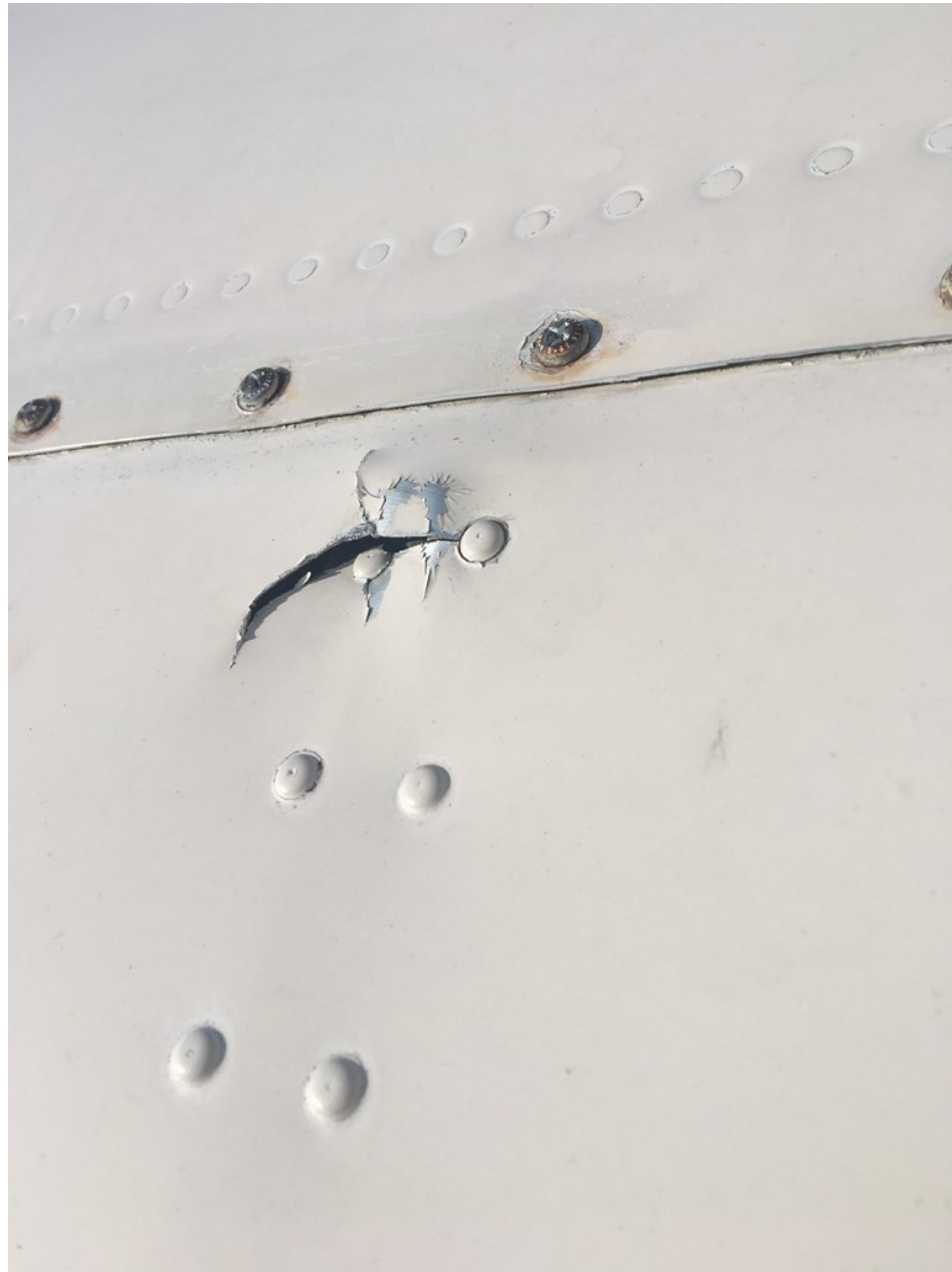
Photo 3 – Upper Left Wing Tear (Photo Courtesy of FAA)
