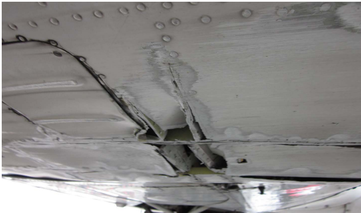
Figure 2 Substantial damage to the ribs and stringers (Photo courtesy of the FAA)
