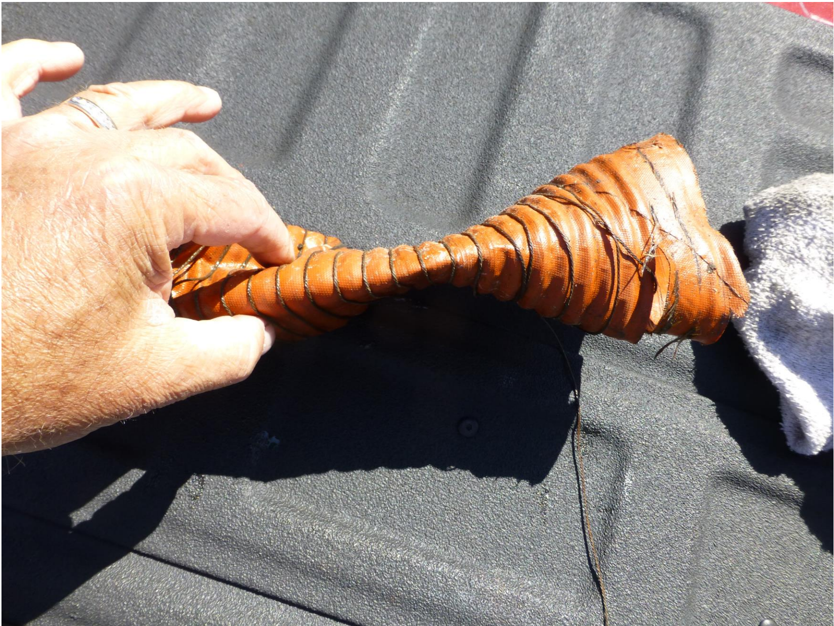
Photo 4 – Side view of collapsed duct-removed
