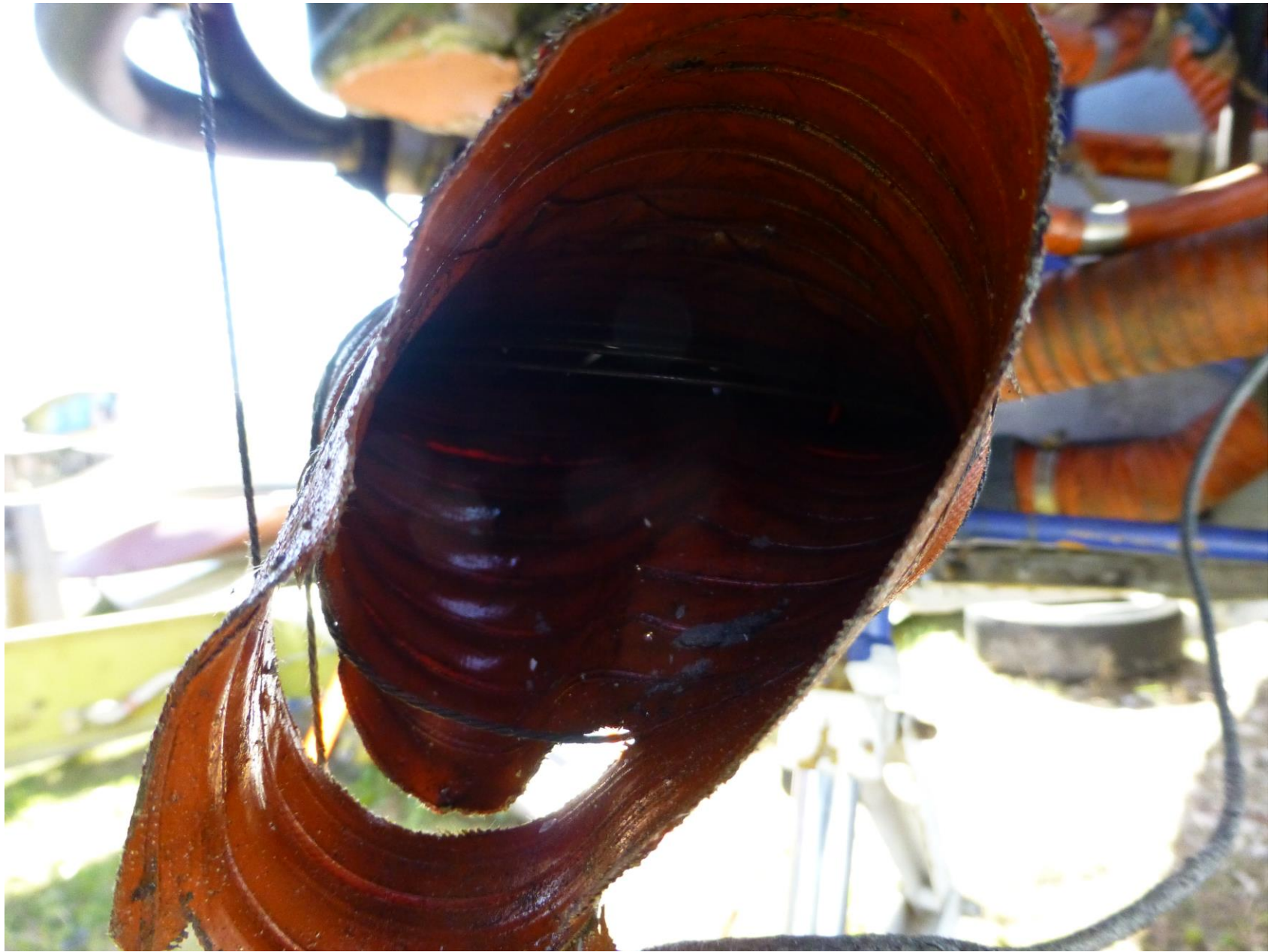
Photo 3 – View down collapsed duct
