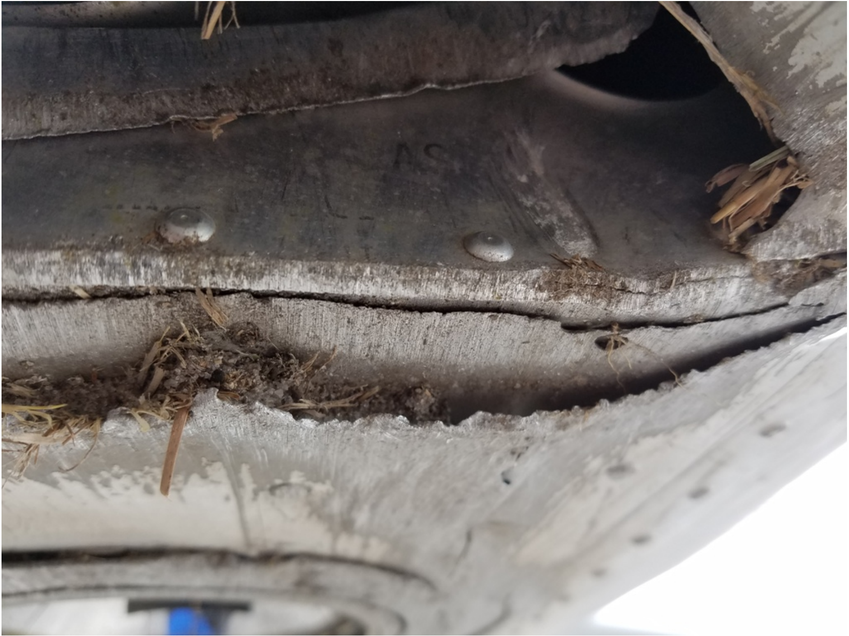
Photo 3 – Left Spar Damage (Photo Courtesy of FAA)
