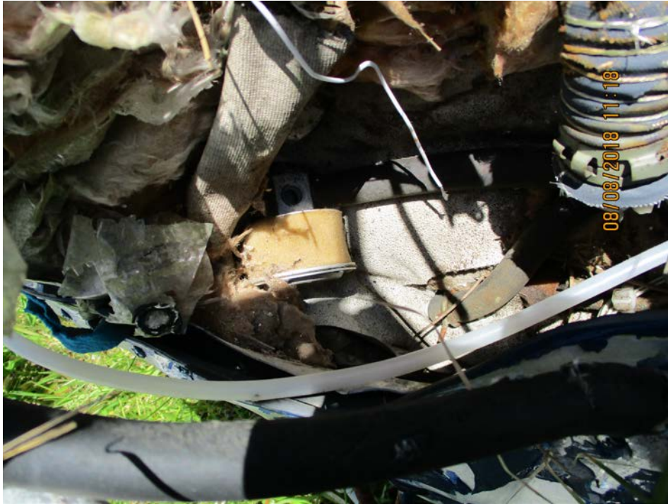
Photo 3. Vacuum regulating valve.
