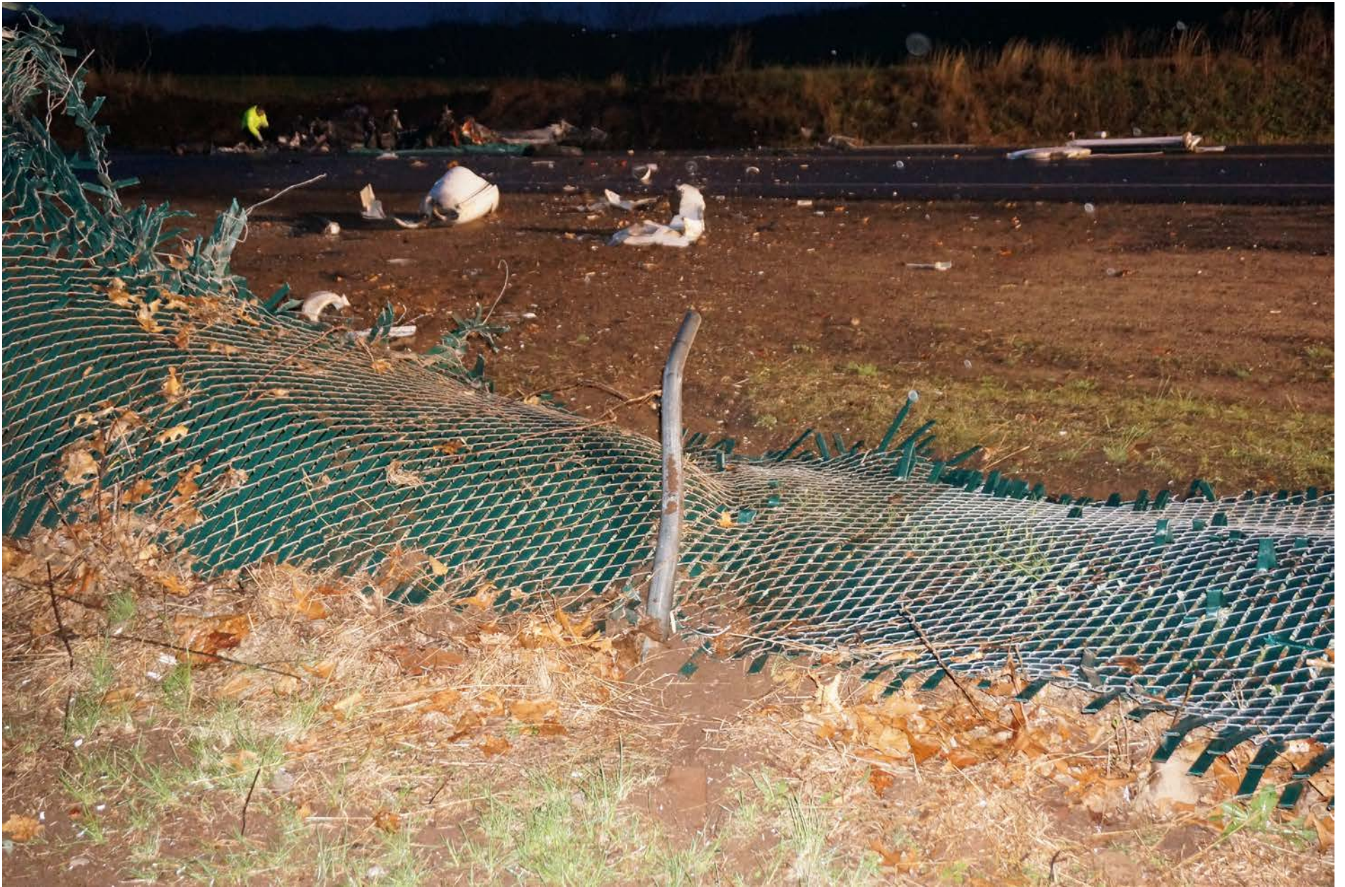
Photo 2 – Close Up Photograph of Breach
