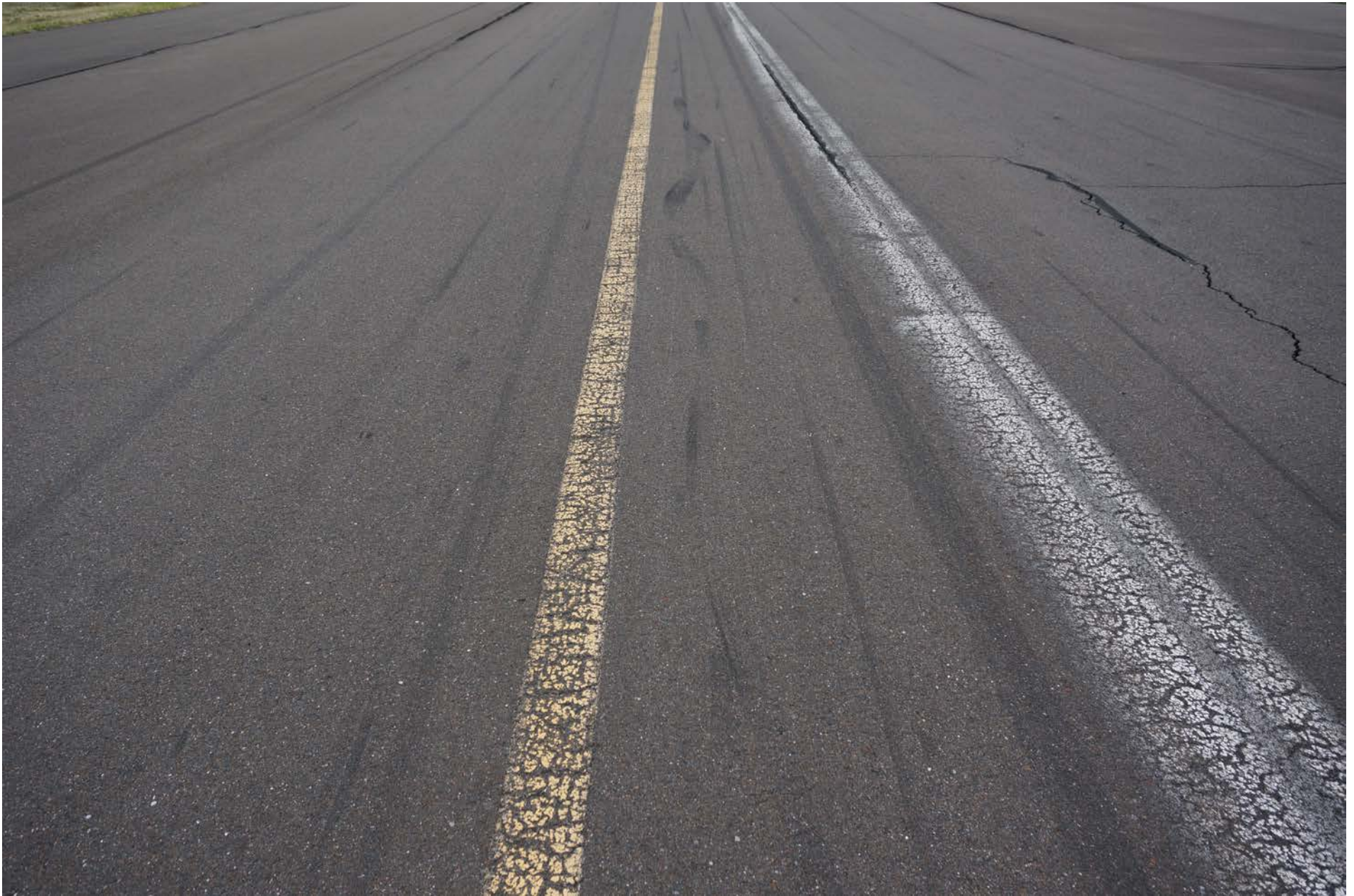
Photo 17 - Second Set of Nose Wheel Tire Marks and Nose Wheel Pant Paint Transfers
