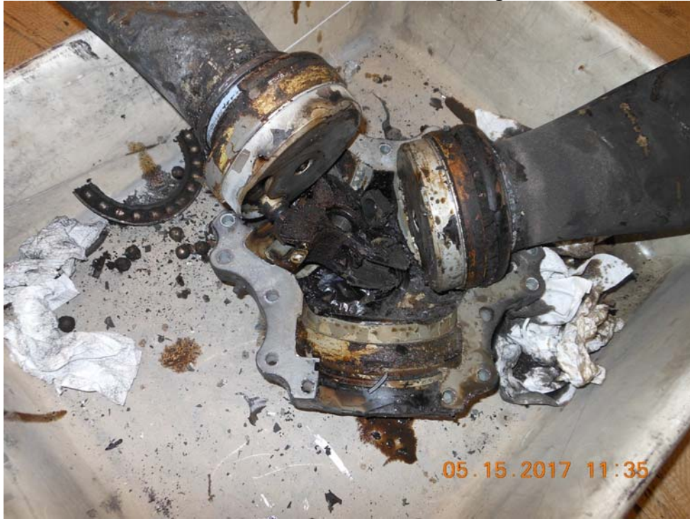
Photo #3 – Internal hub heat damage
