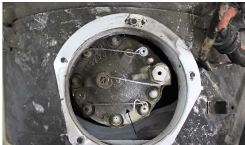
Photo No. 75 Bleed off valve
