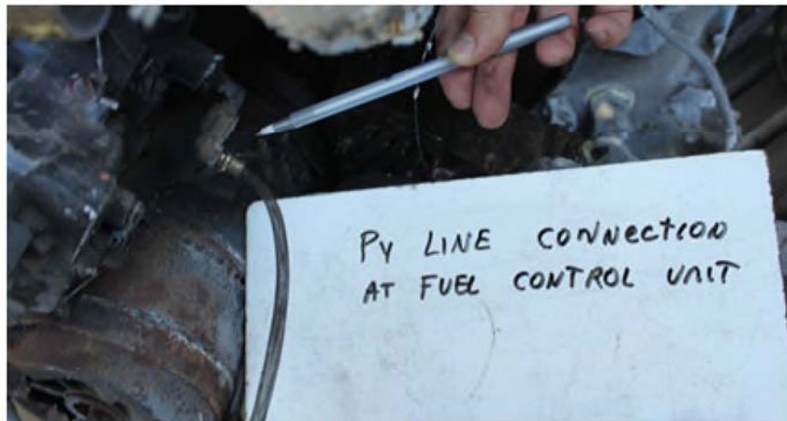
Photo No. 21 Py line at the fuel control unit
