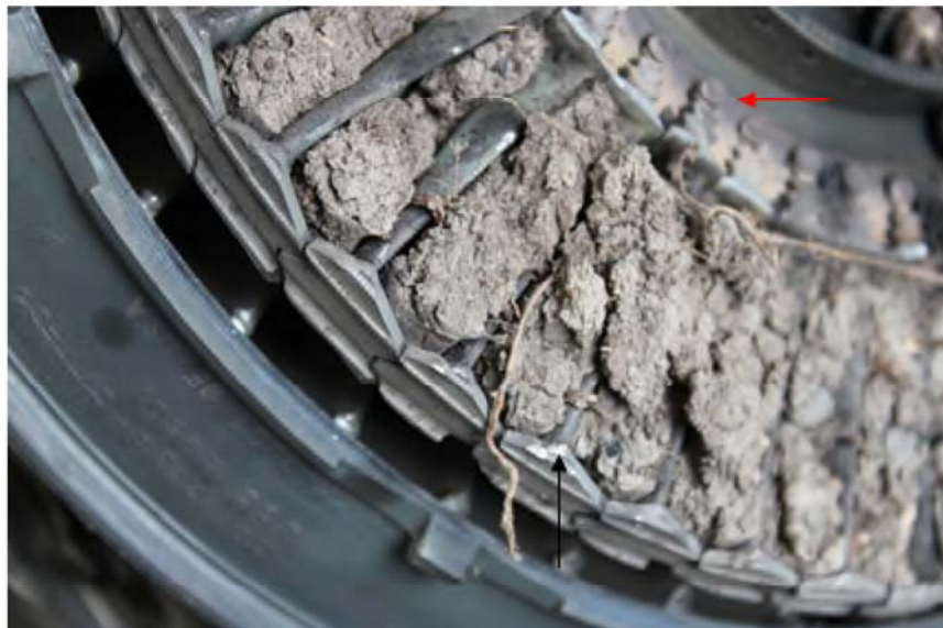
Photo No. 56 Closer view showing first stage power turbine blades displacement
