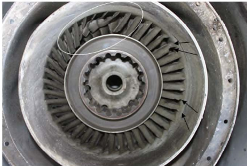
Photo No. 35 First stage stator and shroud
