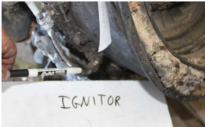
Photo No. 67 One of the ignitor leads at the gas generator case
