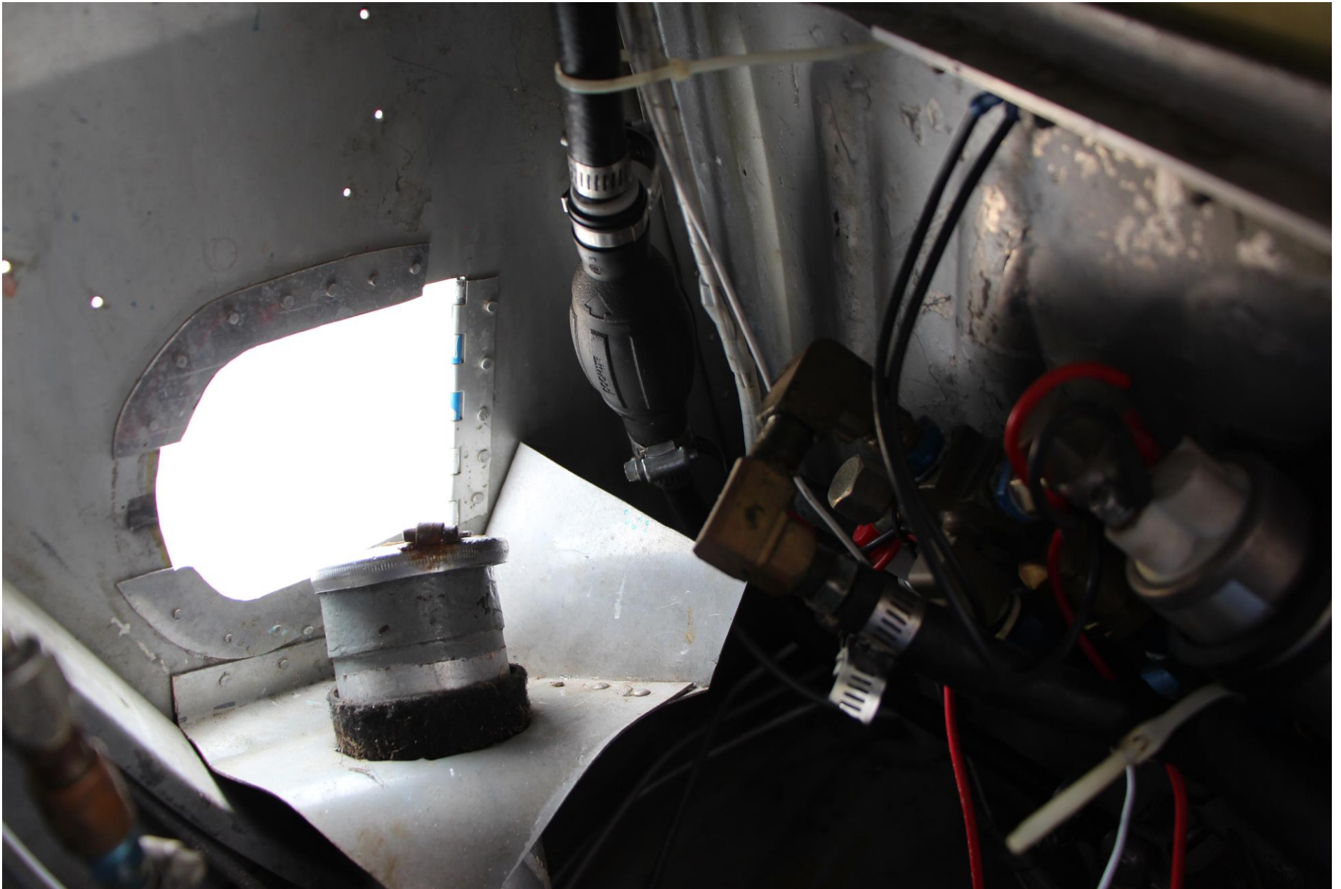
Photo 2 – Unapproved fuel line
