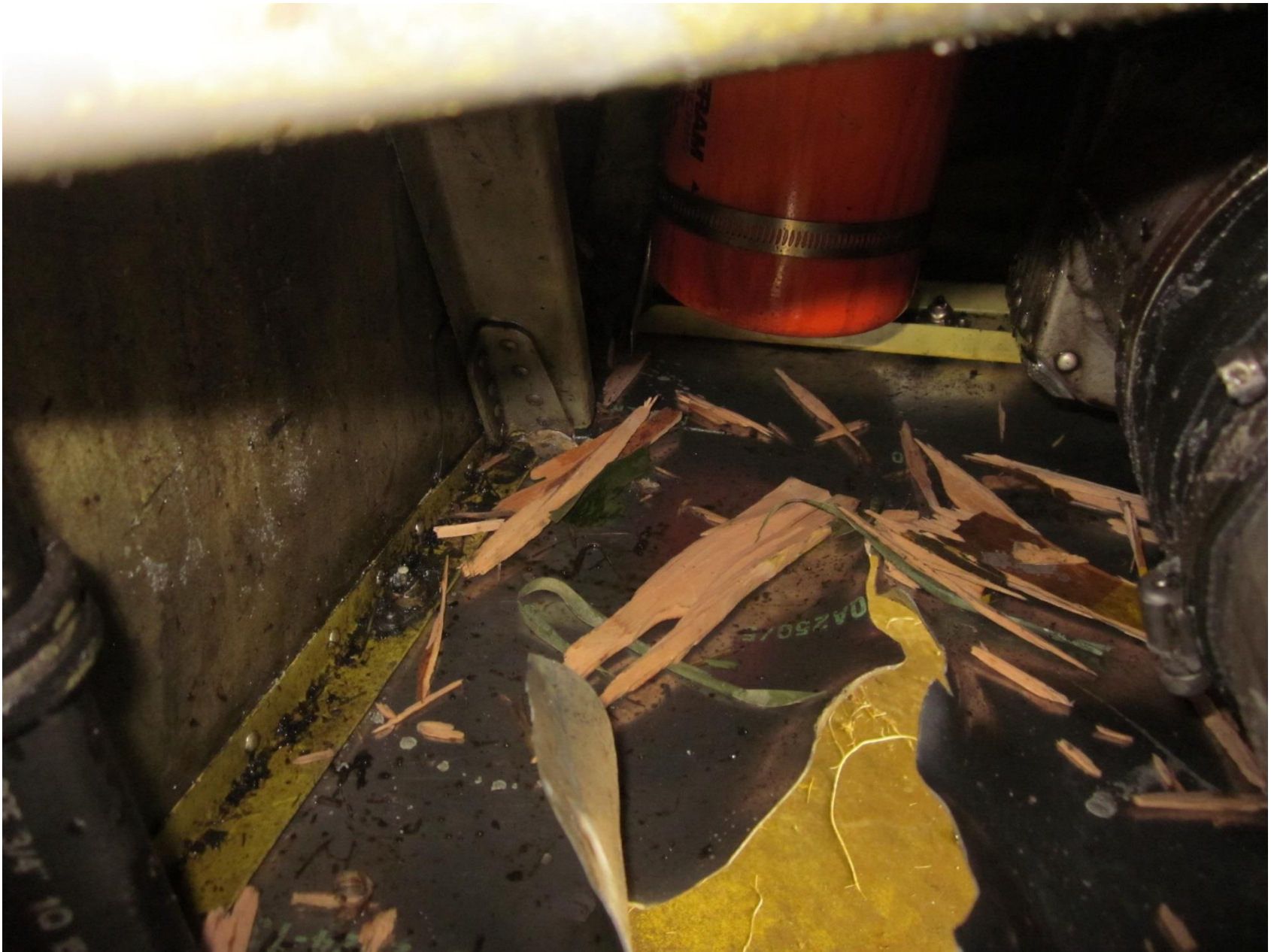
Photo 4 – Splintered Spray Pump Blade Sections (FAA Photo)
