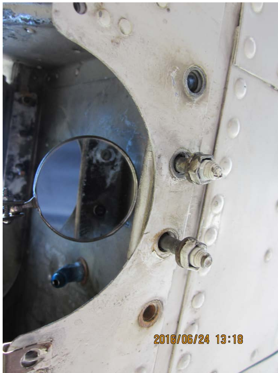
Photo 3 – FAA photo-View of spar damage
