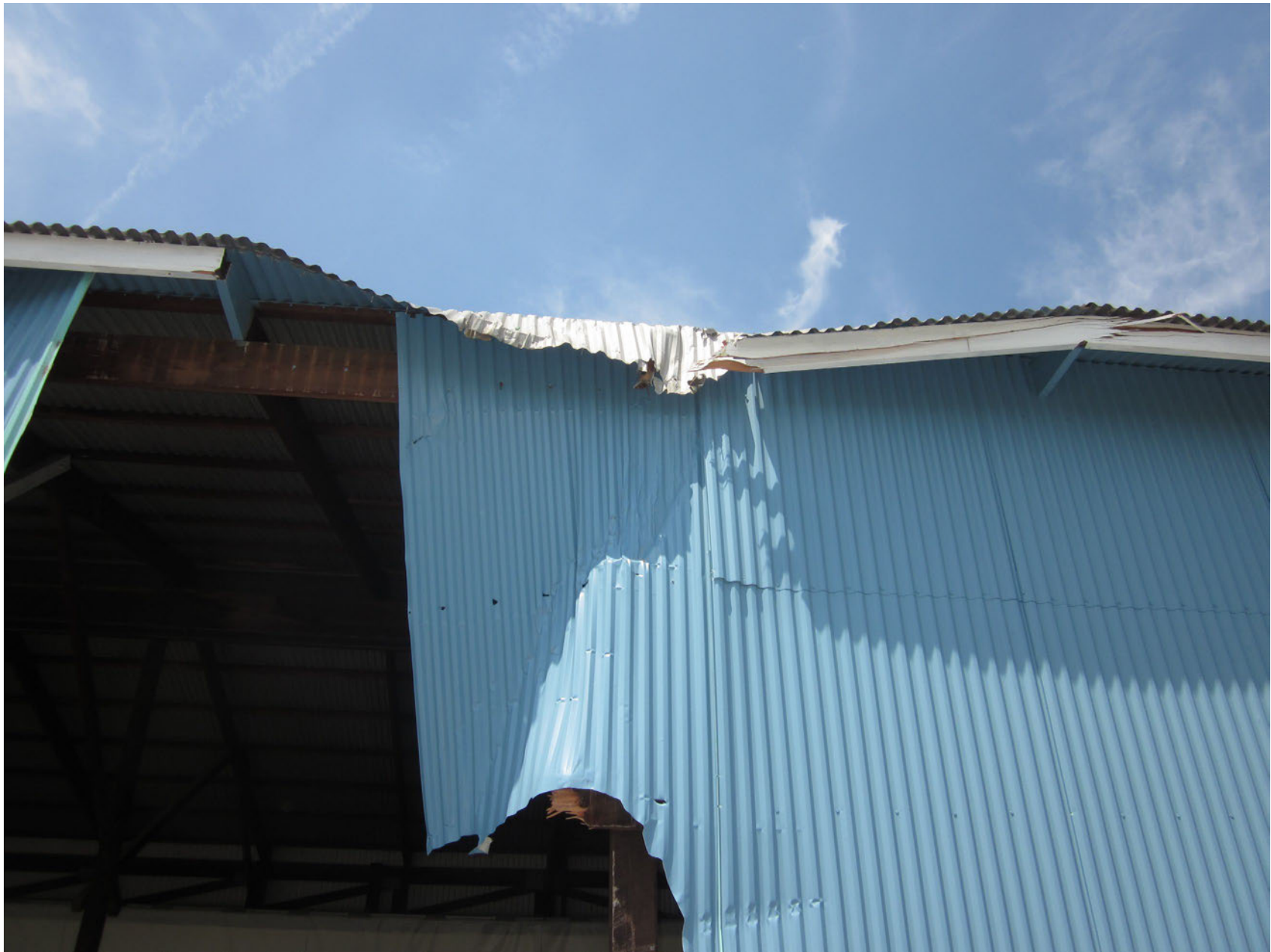
Photo 3 - Close Up of Upper Area of Impact Point with Hangar – Courtesy of FAA
