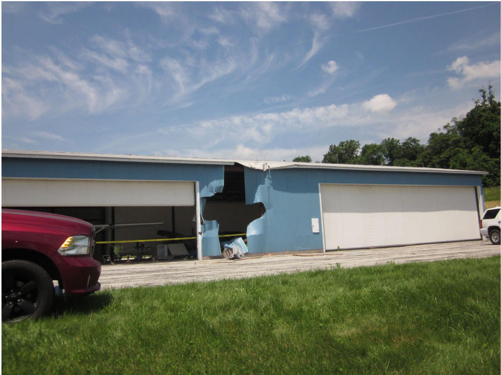
Photo 1 – Impact Point with Hangar – Courtesy of FAA
