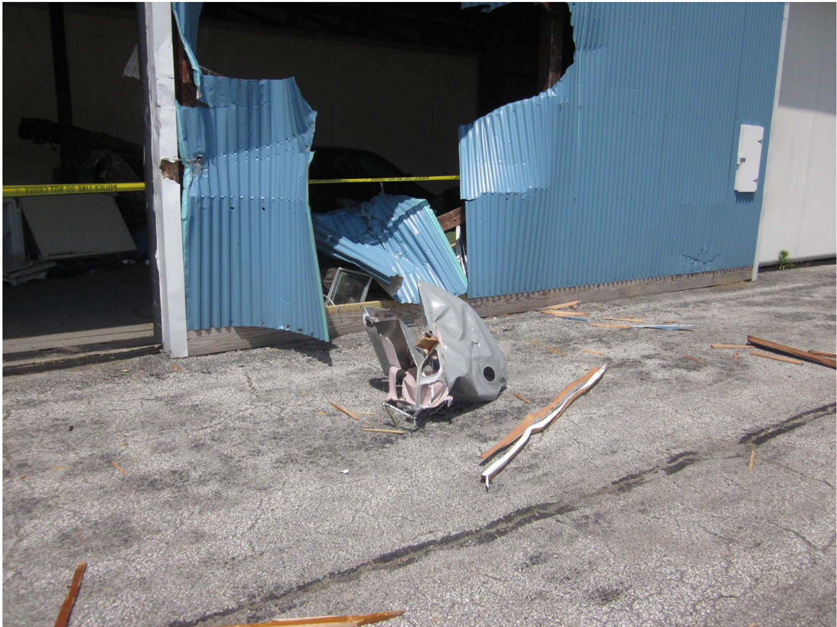
Photo 2 – Close up of Lower Area of Impact Point with Hangar – Courtesy of FAA
