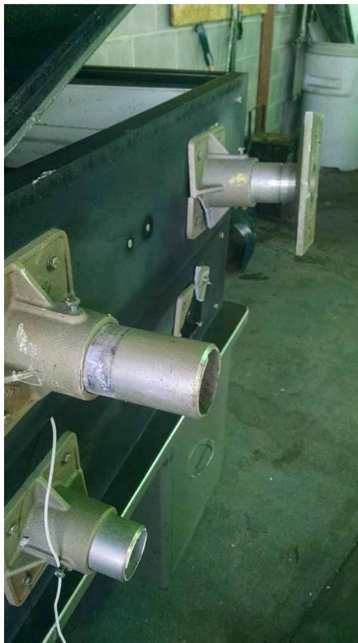
Photo 7 - FAA Digital Photograph. View Depicting Both Damaged Signs. Note the 2 fractured Frangible Posts in the Foreground.
