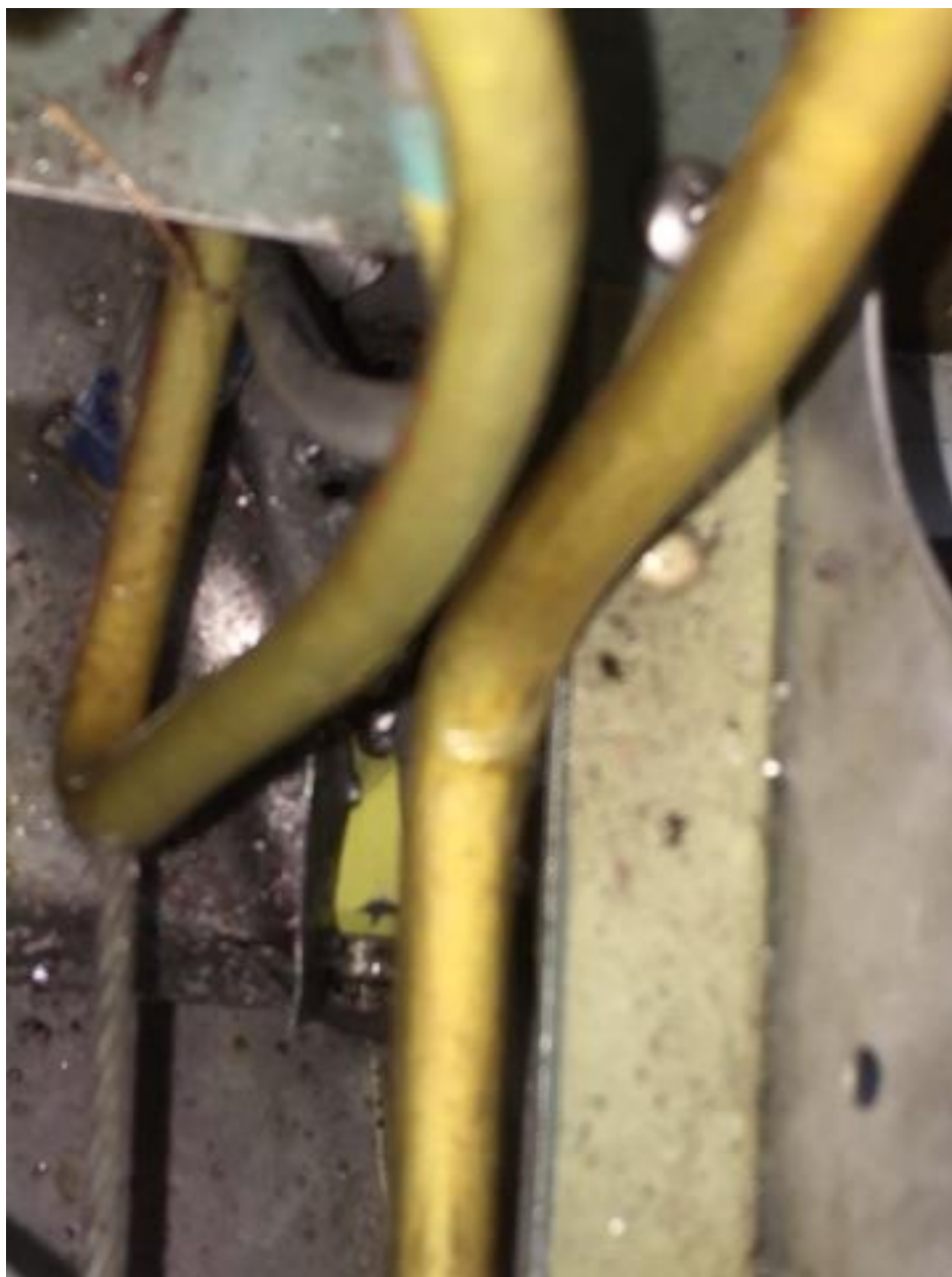
Photo 3 – Structural Damage (FAA Photo)
