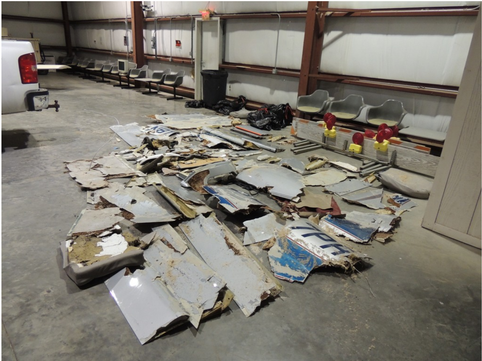
Photo 2 – Airplane Debris on Hangar Floor (Provided by FAA)
