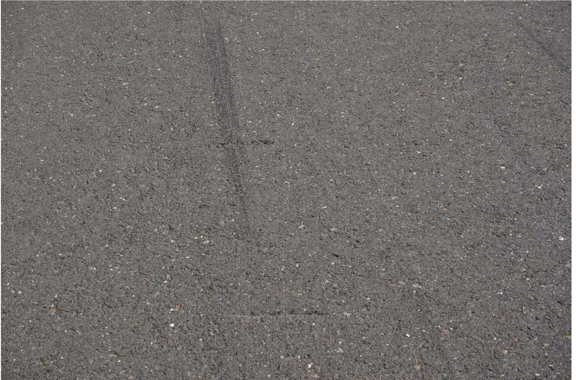
Photo 19 – Close Up of Tire Mark on Runway
