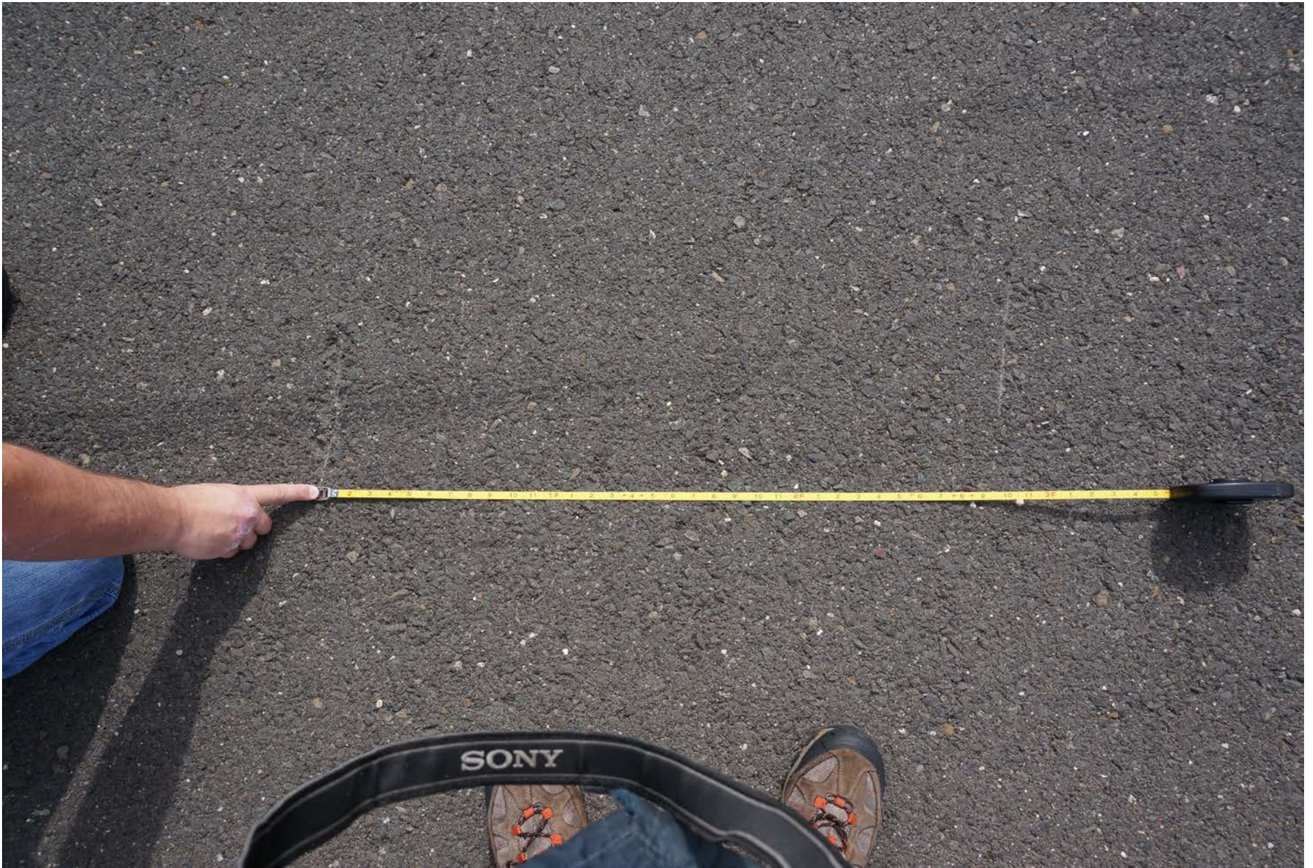
Photo 16 – Propeller Strike Marks on Runway
