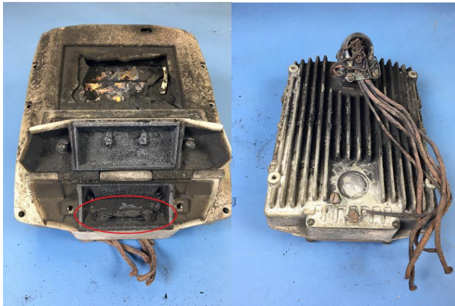
Figure 1. Photo of damaged unit
