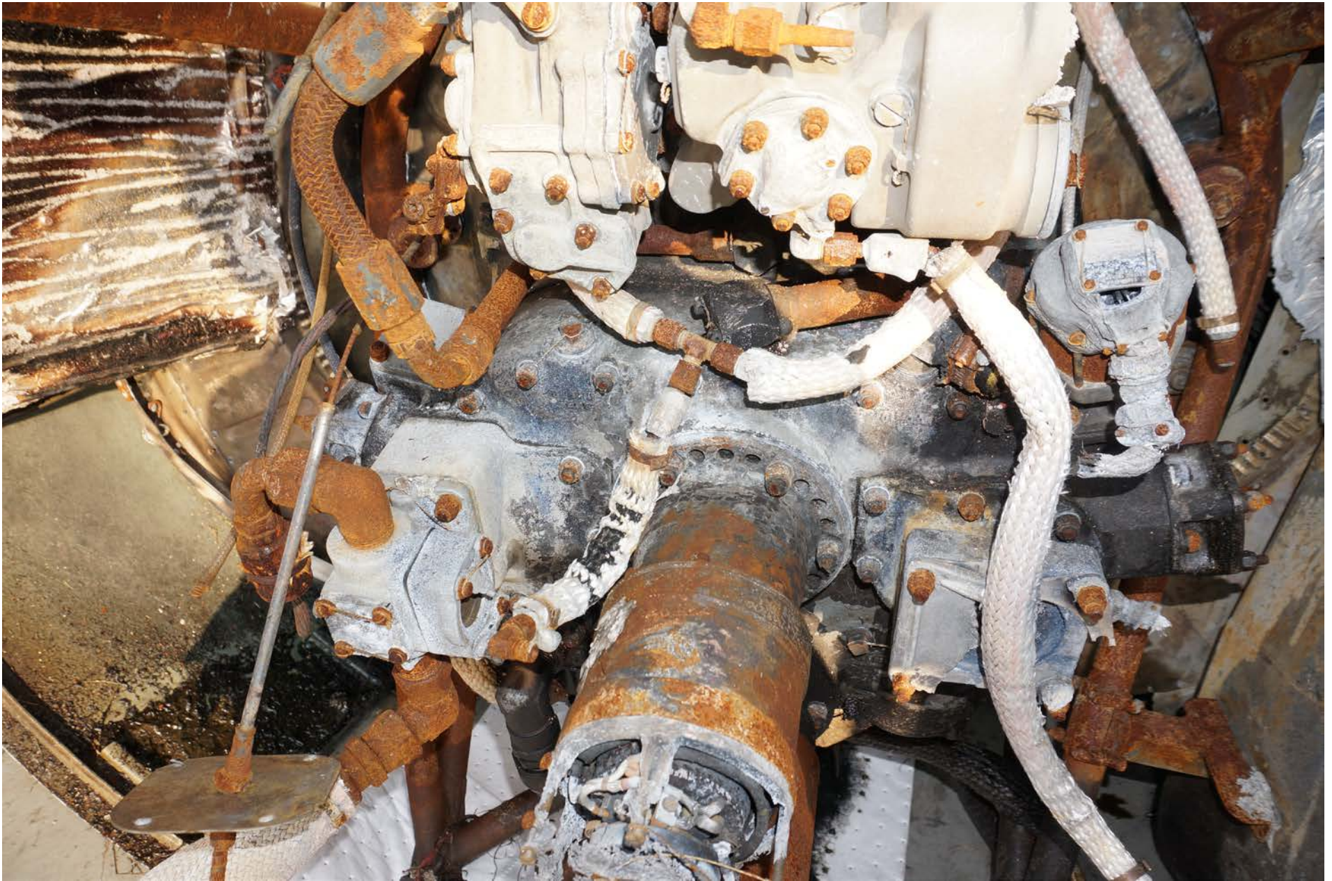
Photo 18 – Close Up of Fire Sleeved Hoses
