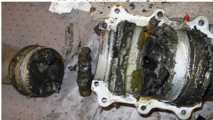
Photo #5 – Over-servicing with grease
