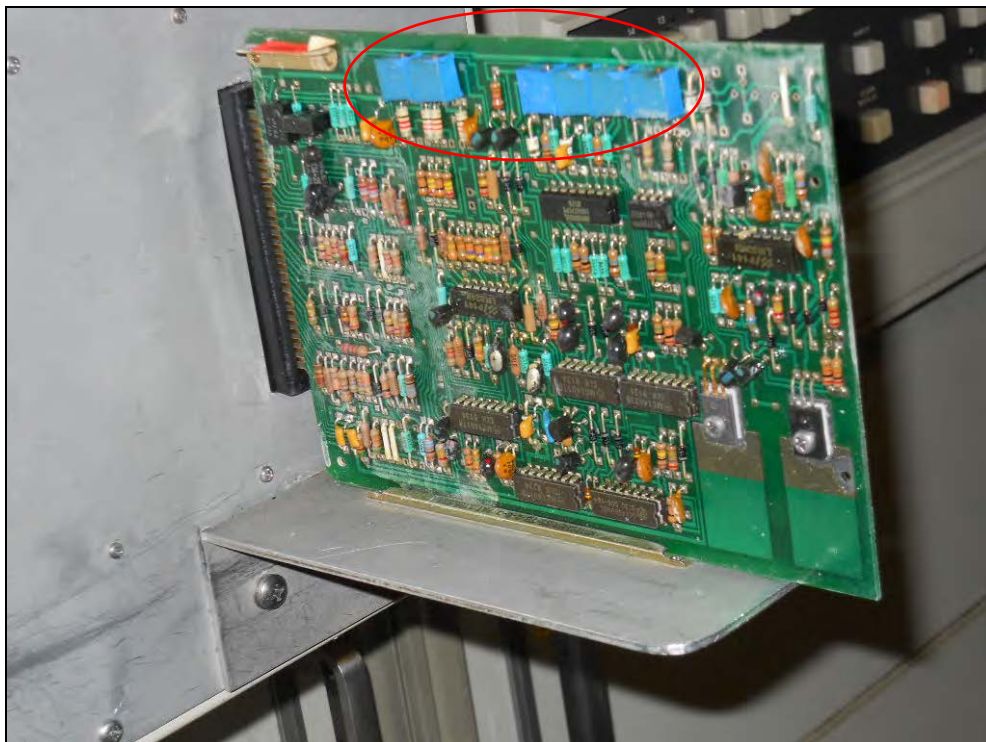
The six potentiometers were not adjusted during ATE testing to preserve post-accident condition
