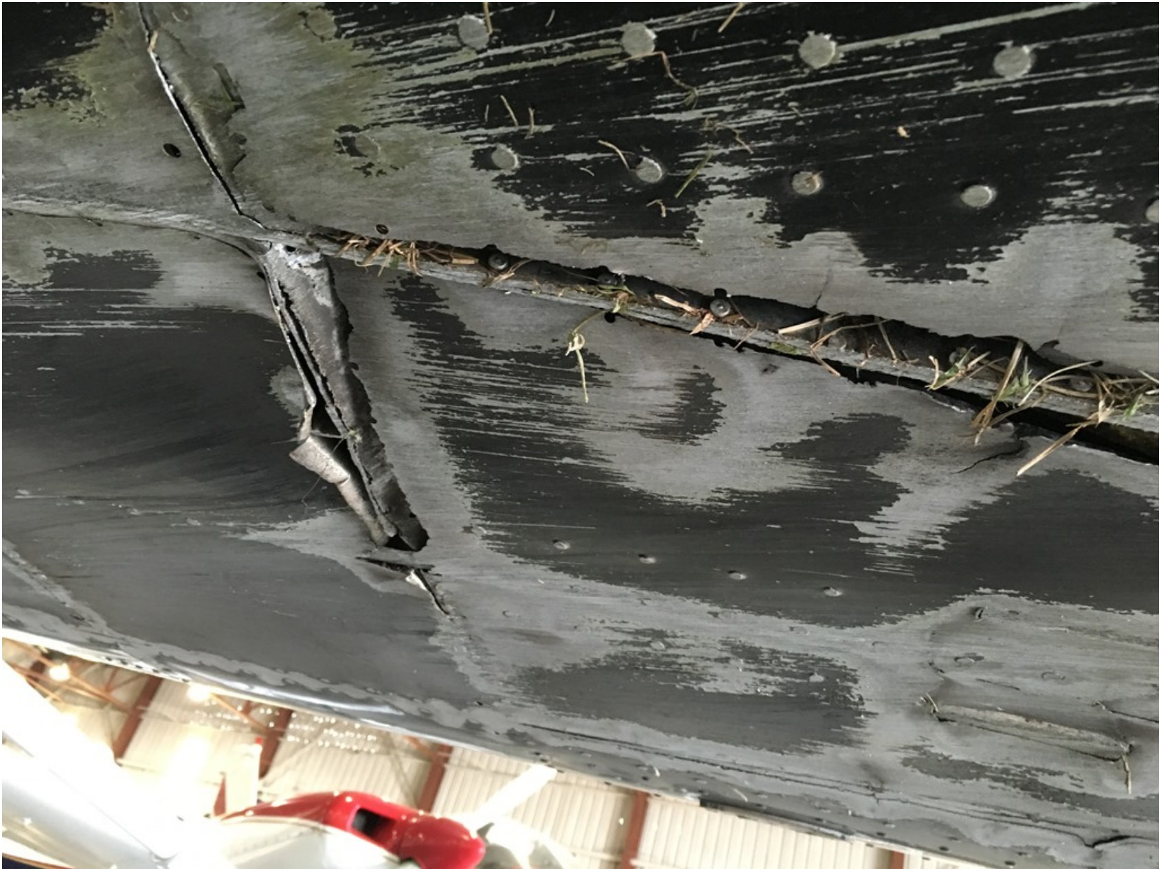
Photo 2 – Lower Fuselage Damage
