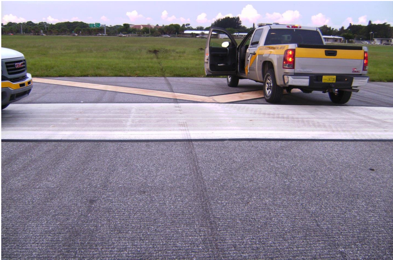
Figure 4 Skid marks leading off the runway
