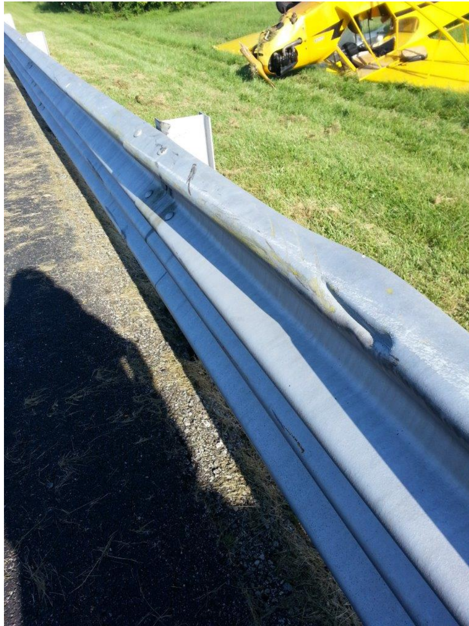
Photo 2 – View of Guardrail Damage facing Direction of Travel (WVSP)
