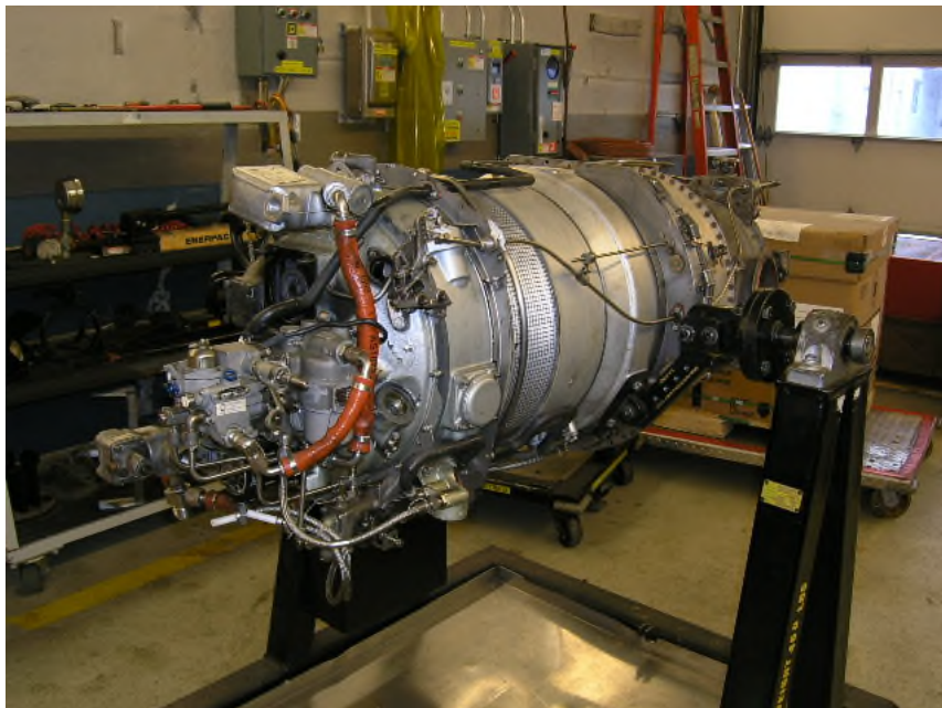
Photo No. 4 Engine right hand aft view.
