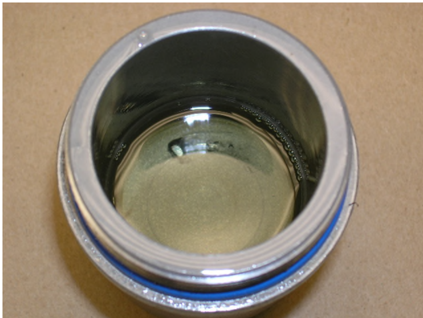
Photo No. 12 Fuel filter housing and residual fuel.
