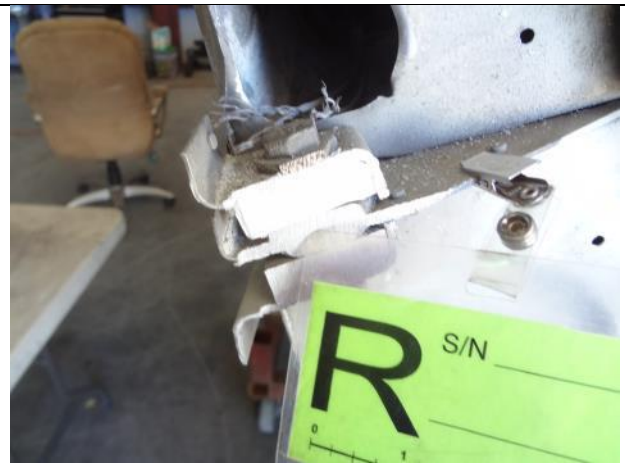
Photo 12: Right Wing Flight Control Cable with Recovery Cut Marks
