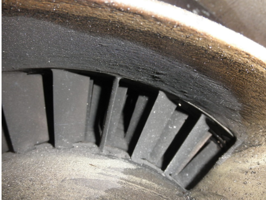
Photo No. 10: Close up view of high pressure compressor inlet guide vanes and 1st stage blades.
