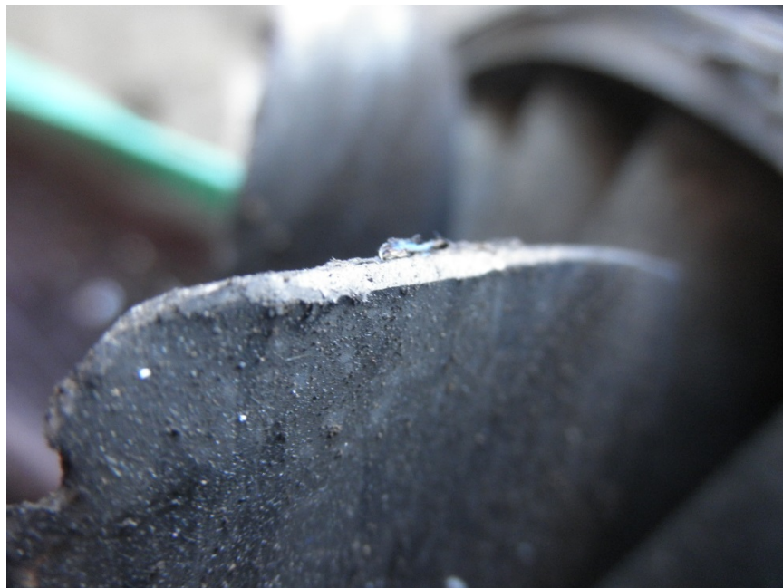
Photo No. 5: Close up of 1st stage fan blade tip showing flat spot on concave corner.
