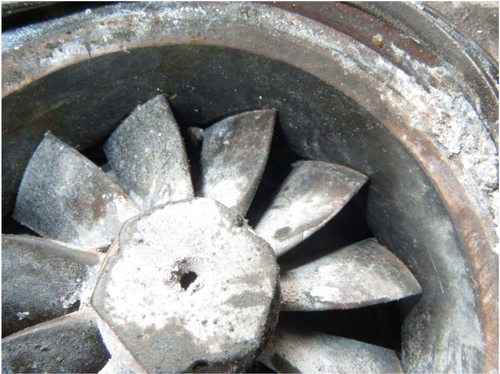
Photo 7 – Close Up of Turbine Wheel
