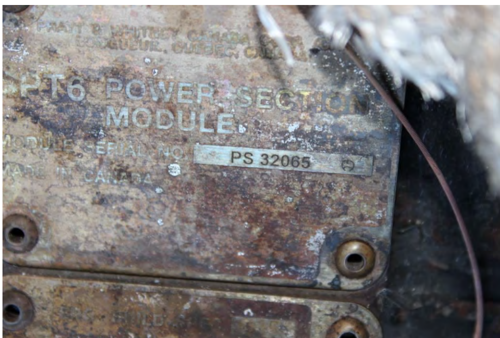
Photo No. 99, View of the power section data plate
