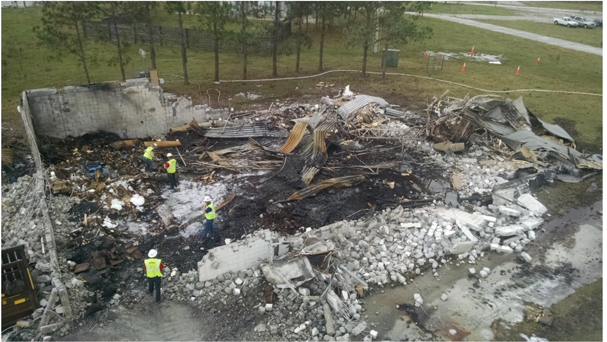
Photo 3 - Digital Photograph Taken by Fire Rescue. View Taken from Fire Rescue Ladder Depicting the Impacted Building.
