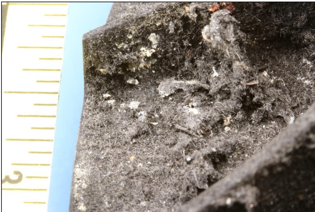
Figure 2. Close view of charred debris on the centrifugal compressor.
