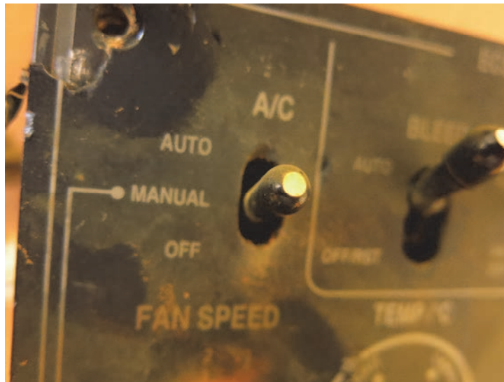
Figure 52. The AC switch toggle had recessed into the panel and was loose. The impact position was indeterminate.
