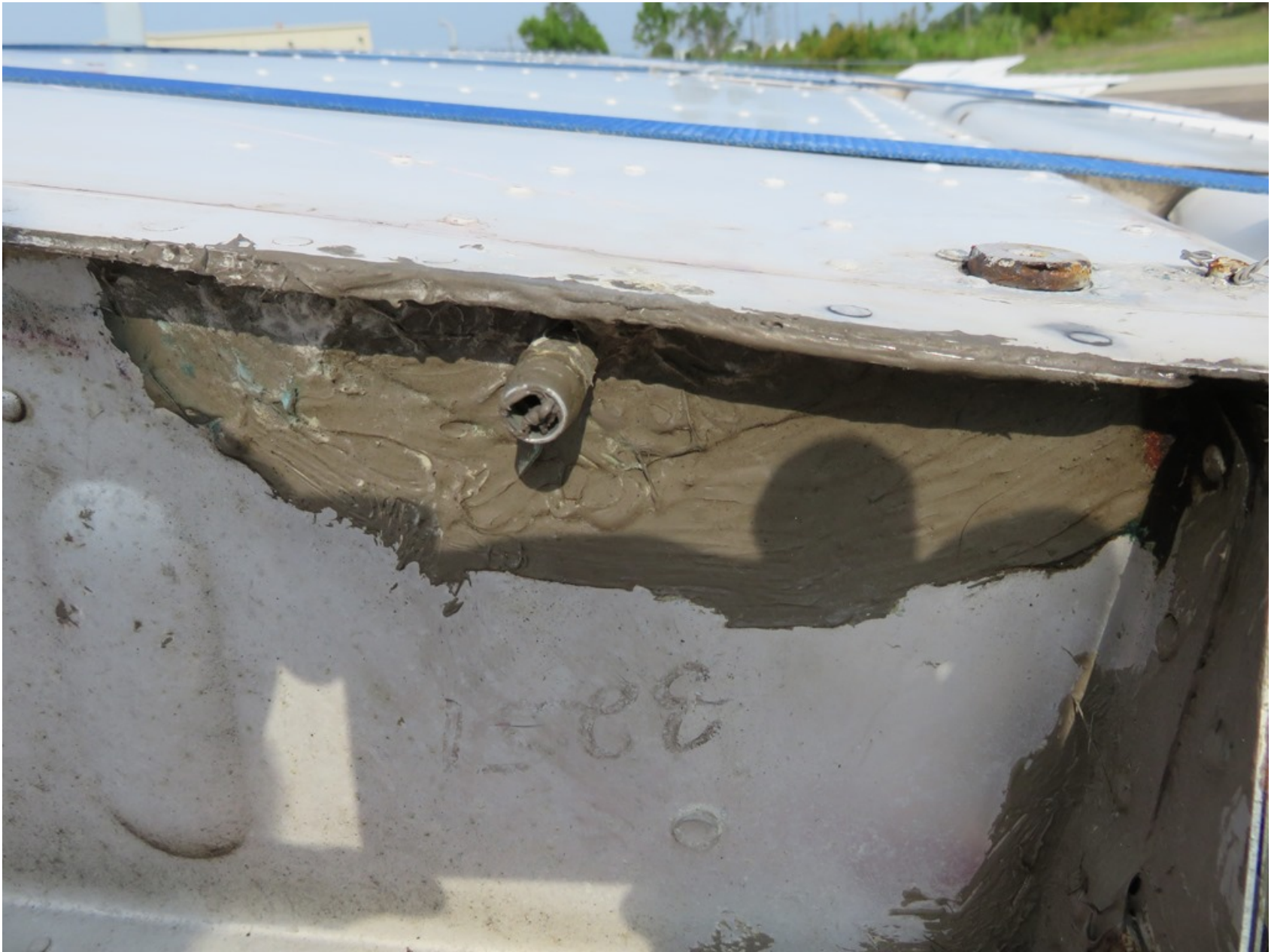
Photo 6 – View of Sealant in Left Wing Fuel Line
