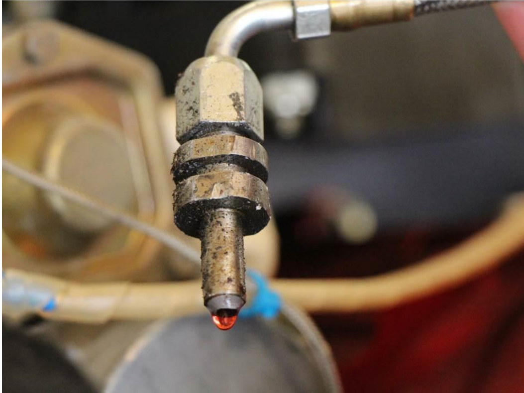
Photo 2 -The propeller hydraulic line fitting is designed to fracture if the slave piston starts rotating with the propeller. The fitting at the end of the inflow tube was broken, which allowed the hydraulic fluid to escape and also allowed the slave servo to rotate with the propeller rather than remaining stationary with the engine. In addition, the blades could rotate to a lesser pitch angle.
