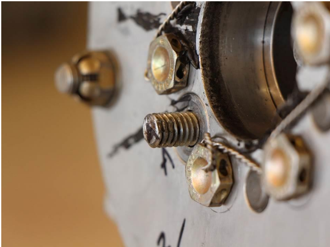
Photo 7 - Damage to the fine pitch adjusting bolt (A).
