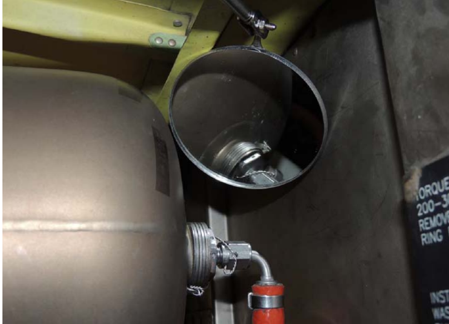
Outer Combustion Case (Sheet Metal and Weld Seams) - Inspection FIG. 1
