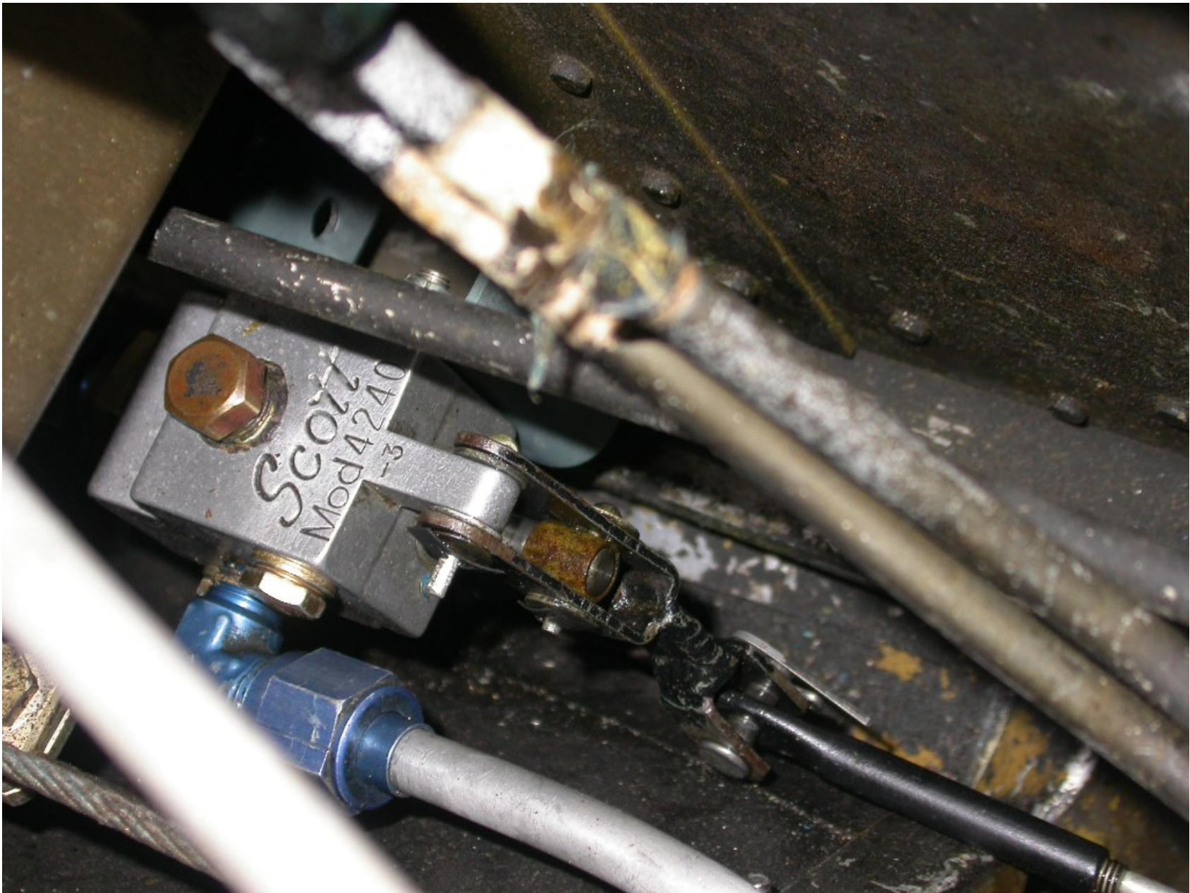
Photo 9 - Right Auxiliary and Main Shutoff Assembly Missing Control Cable
