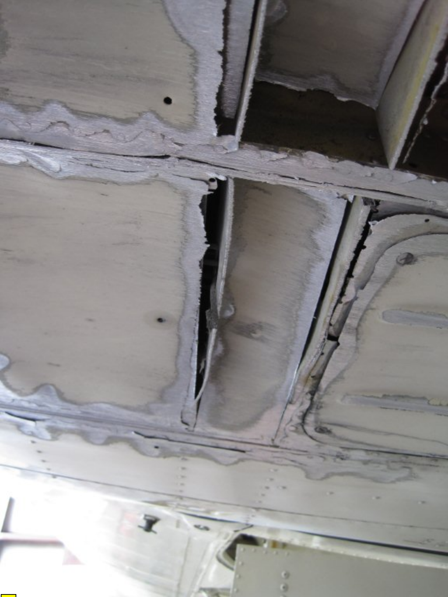
Photo 2: Damage to Airframe Structure (FAA)
