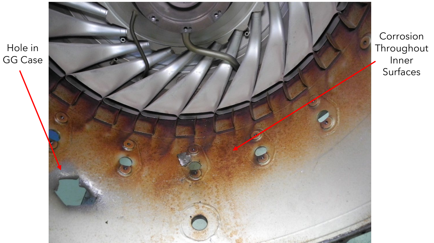
Photo 22 - Hole in GG Case - Inside View
