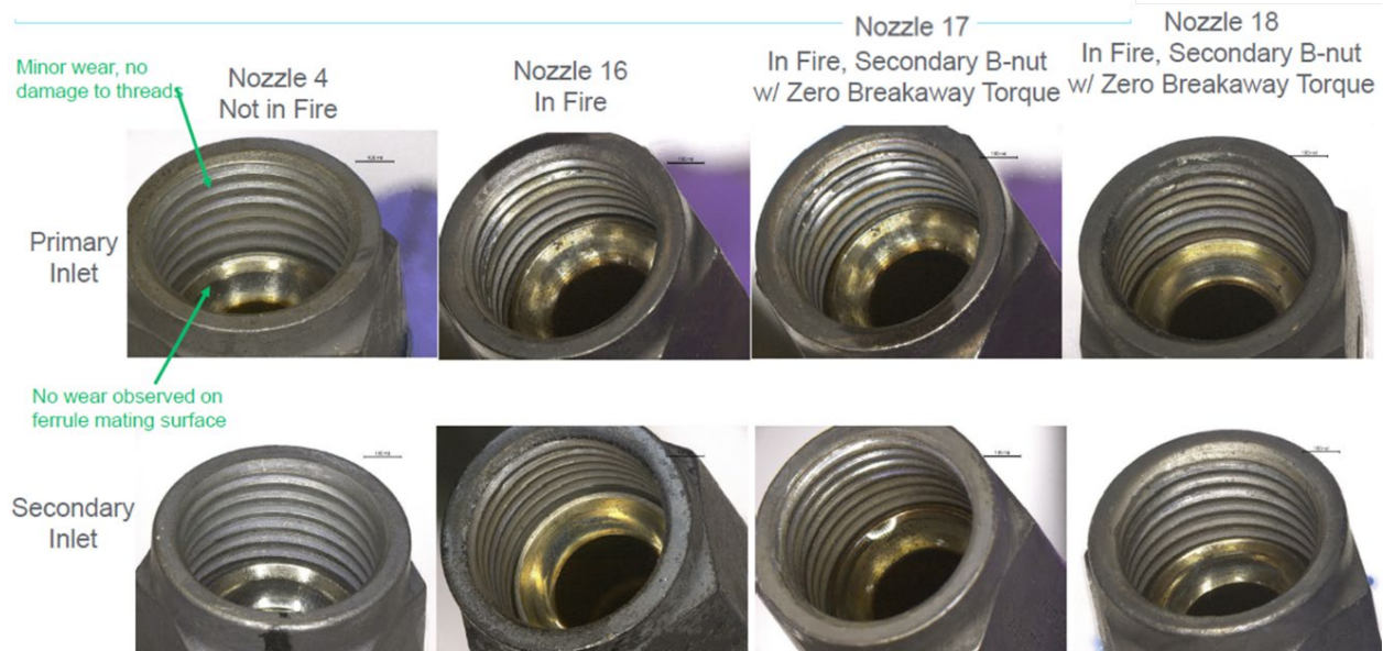
Photo 14- Fuel Nozzles 4, 16, 17, and 18 Primary and Secondary Inlet Threads
