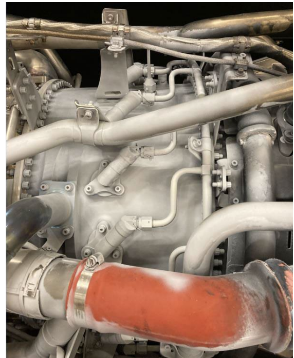
PHOTO 4: FUEL LEAK CHECK WITH DEVELOPER
