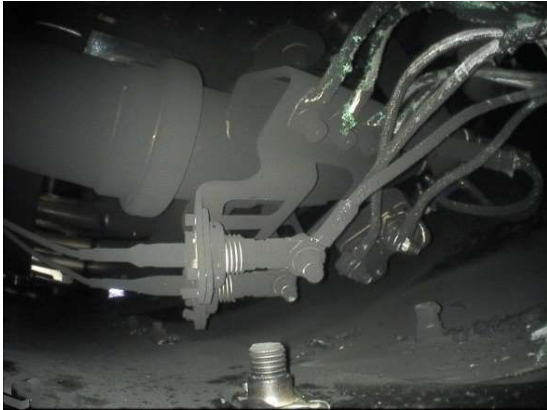
PHOTO 8: CORE FIRE HARNESS THERMALLY DAMAGE (6:00-7:00 O'CLOCK POSITION ALF)
