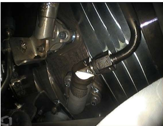
PHOTO 12: FUEL MANIFOLD B-NUT WETTED (6:00-7:00 O'CLOCK POSITION ALF)
