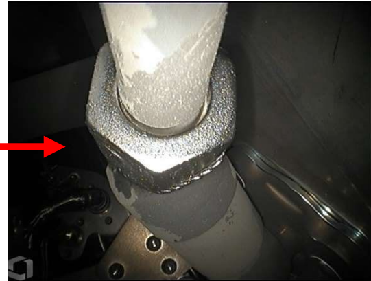
PHOTO 11: FUEL MANIFOLD B-NUT WETTED (12:00-1:00 O'CLOCK POSITION ALF)
