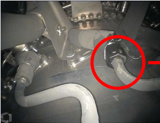
PHOTO 10: FUEL MANIFOLD B-NUT WETTED (12:00-1:00 O'CLOCK POSITION ALF)
