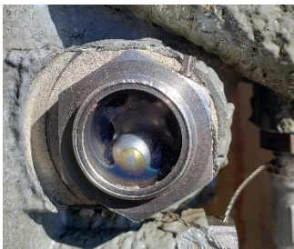
PHOTO 15: OIL TANK SIGHT GAGE
