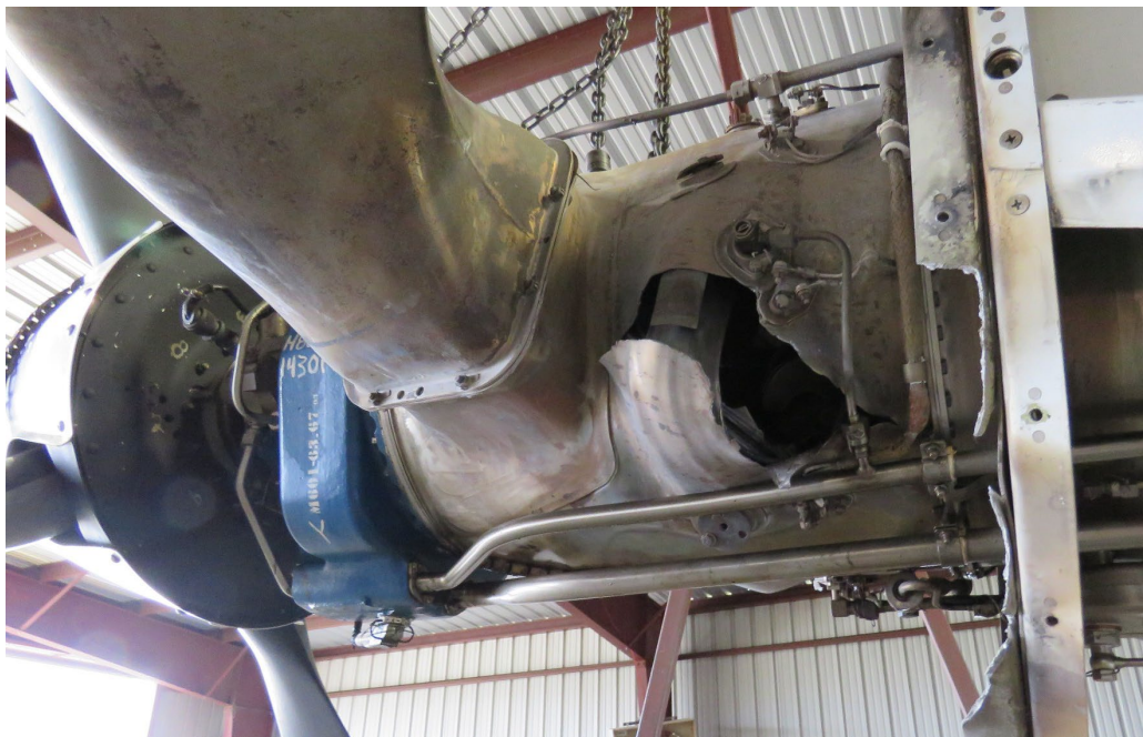
Photo 2: Hole Seen in Left-Hand Side of Engine after Engine Cowl Removal
